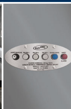
Remote control in the cabin
