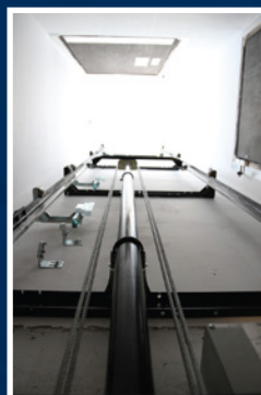
Elevator rails on a wooden wall with Gypsum finish
