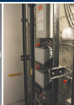
24V mechanism inside the elevator shaft
