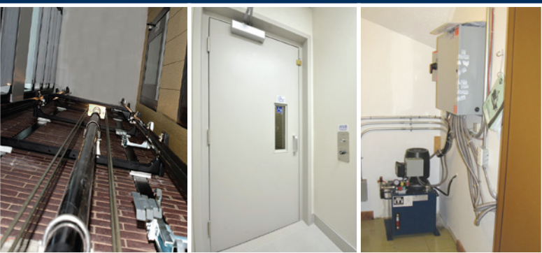
Elevator shaft on concrete wall
